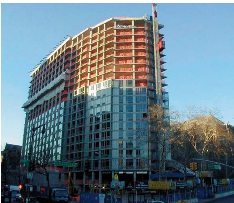
The Avalon Morningside Park apartment building at the southeast corner of the Cathedral campus while under construction. Photo: Cathedral of St. John the Divine
