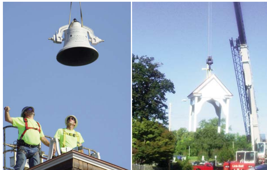
Out of a Blue Sky: Lifting the New Holy Cross Tower into Place.
